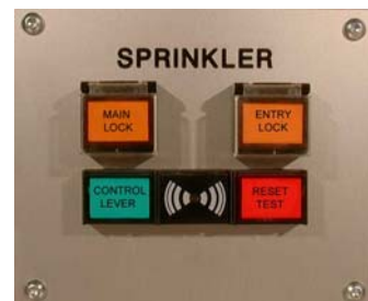
Push buttons for the sprinkler system. Placed in the control system.
