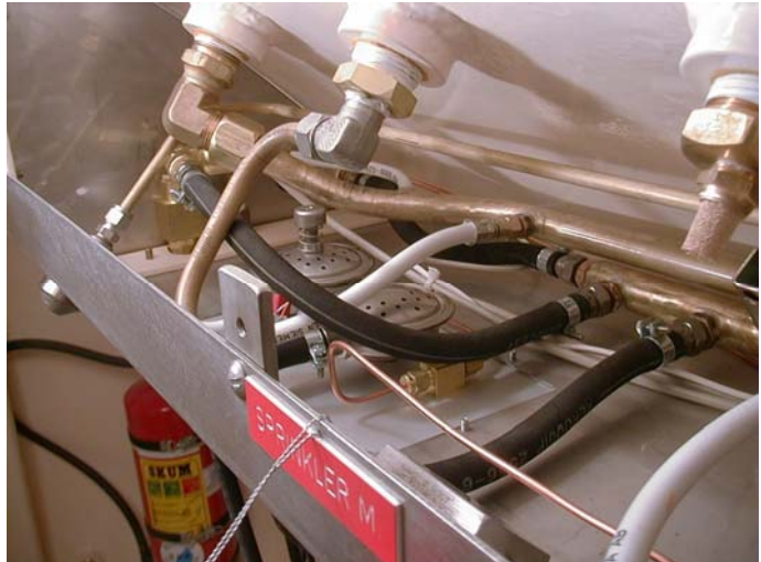
The Sprinkler System built in a control panel.
